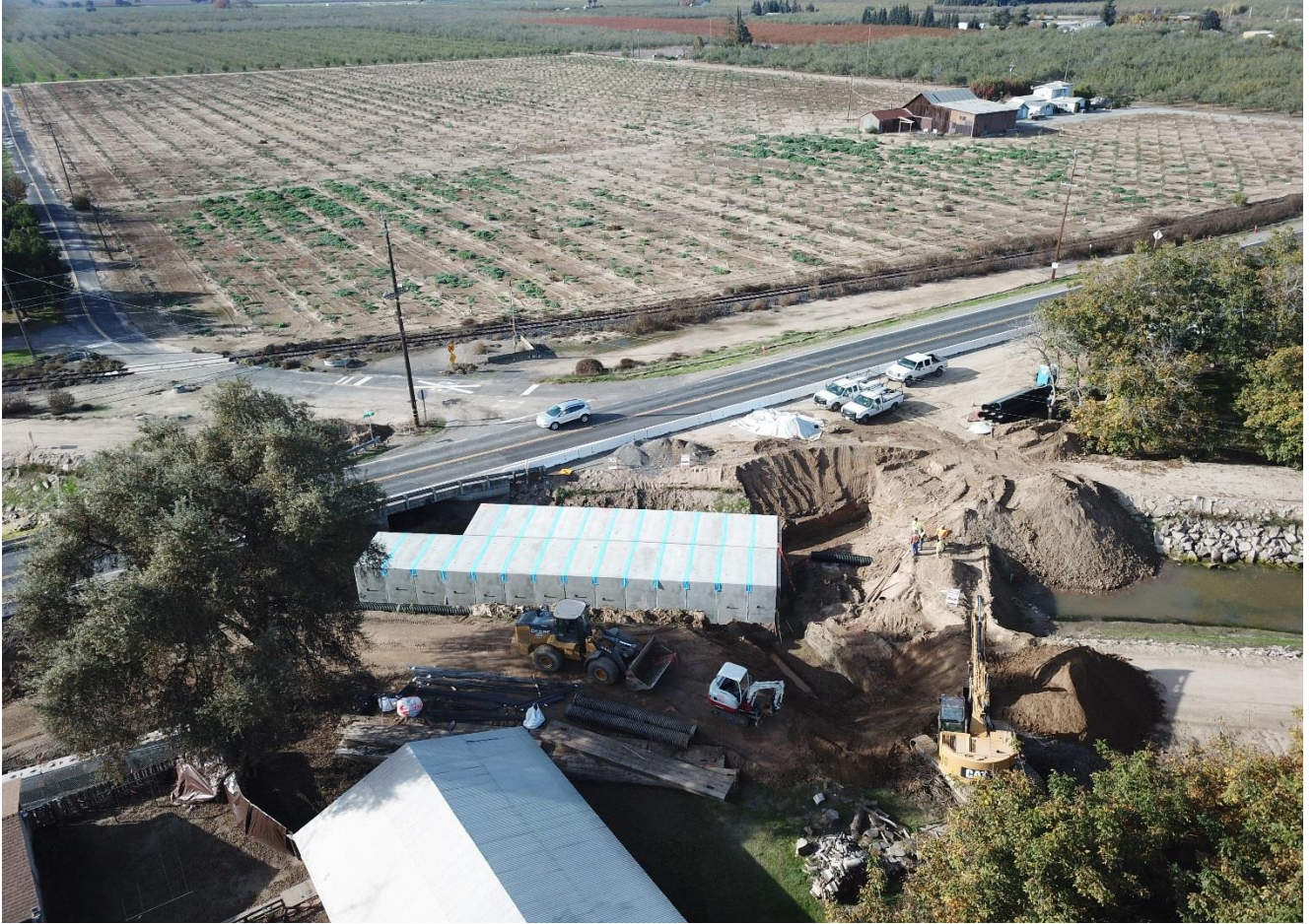
Figure 3: Drone footage of construction progress at McHenry Avenue over the South San Joaquin Irrigation District Canal in the Escalon area. Replacing the existing bridge with a double-box culvert.
