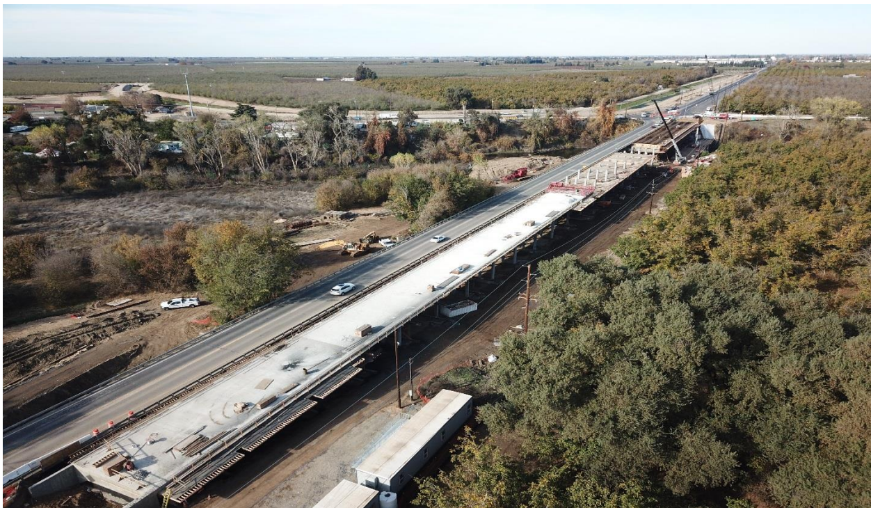
Figure 5: Drone footage of construction progress at McHenry Avenue over the Stanislaus River Bridge in the Escalon Area near the San Joaquin County and Stanislaus County line. Replacing the existing bridge. New east side can be seen adjacent to the existing bridge, which will soon be demolished to construct the west side of the bridge.
