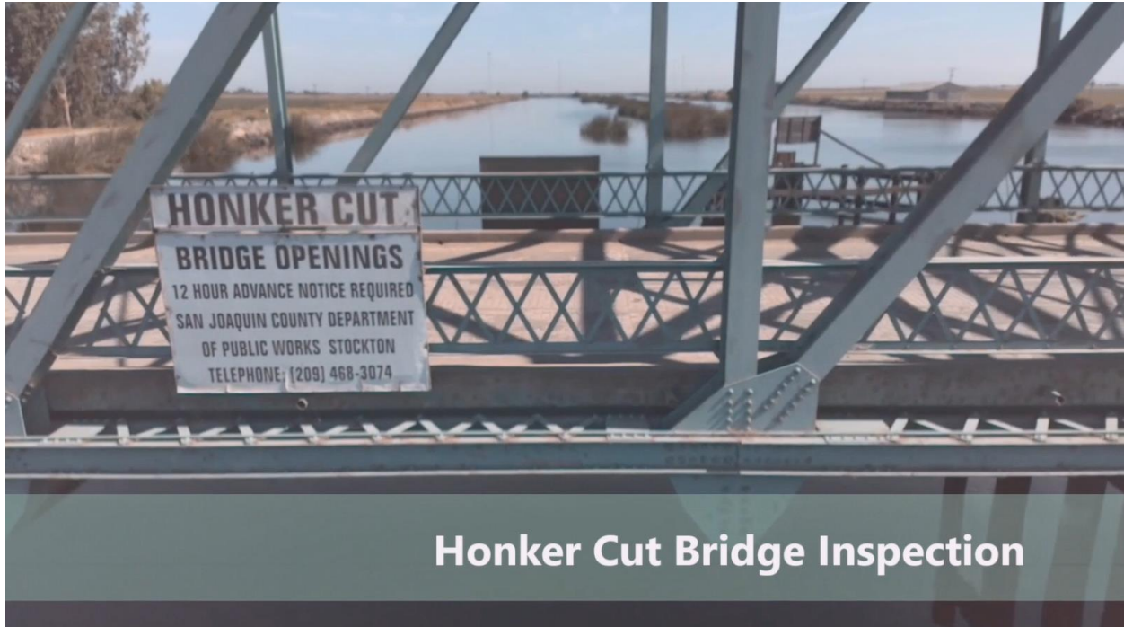
Figure 4: Bridge inspection of structural members at Eight Mile Road over White Slough in the Stockton area.
