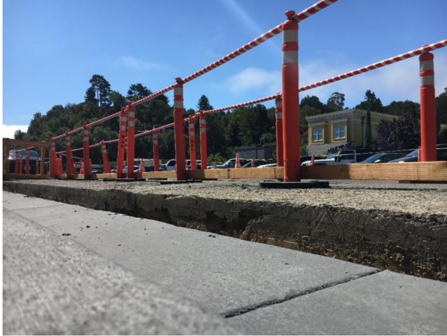
Insufficient Structural Section
