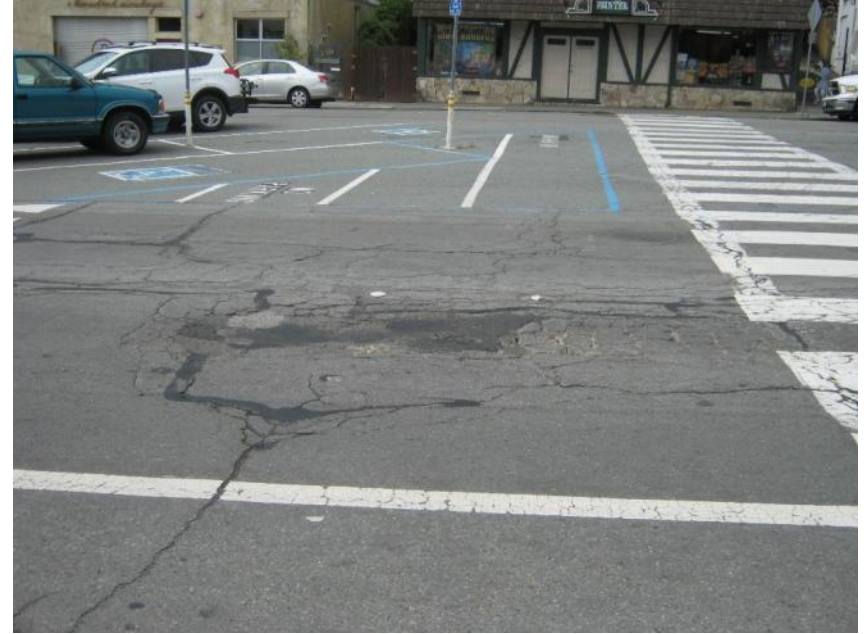
Large Areas of Distress Interim Repairs in 2014 illustrated problem
