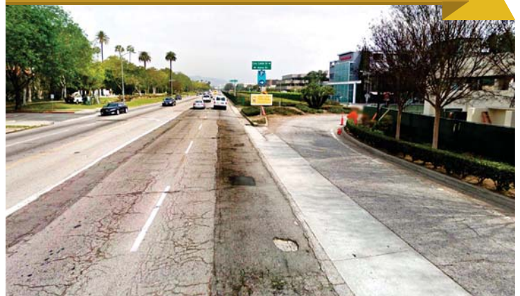
Reconstruction of 1.5 miles of North Santa Monica Boulevard will enhance users' commute and provide a smoother and quieter ride for everyone.
