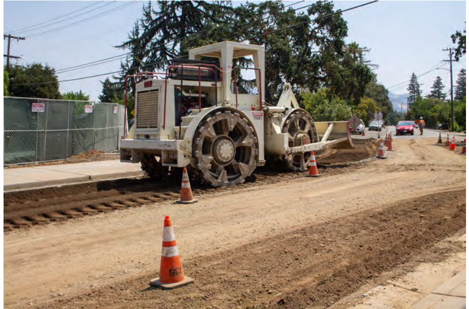
Full Depth Reclamation is a sustainable paving method that grinds up and reuses cement base material to create a stronger, longer-lasting road
