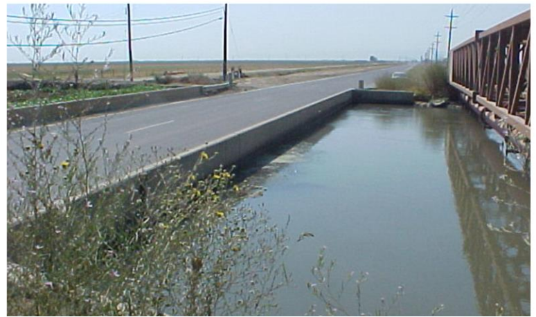
Before: Southward view of the west side of the bridge, which had become submerged.
