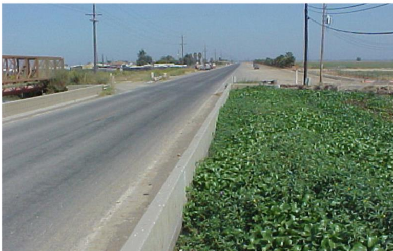
Before: Northward view of the east side of the bridge, showing the effects of subsidence.
