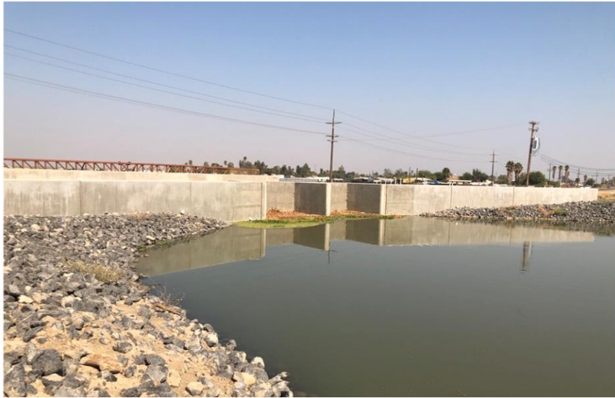
After: East side view of the new double box culvert at high water levels.
