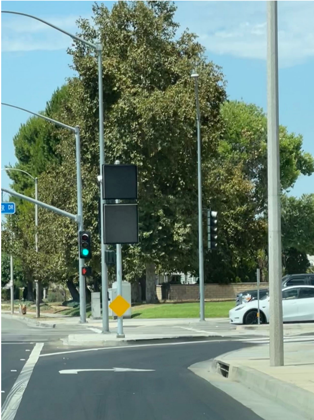
No Pedestrians Present: Active Warning Signage is non-illuminated
