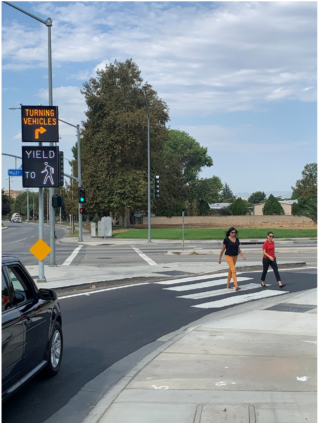
Pedestrians Present: Active Warning Signage is illuminated
