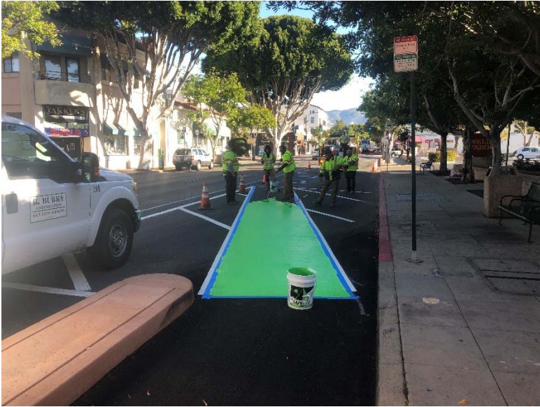
Application of green bike lane
