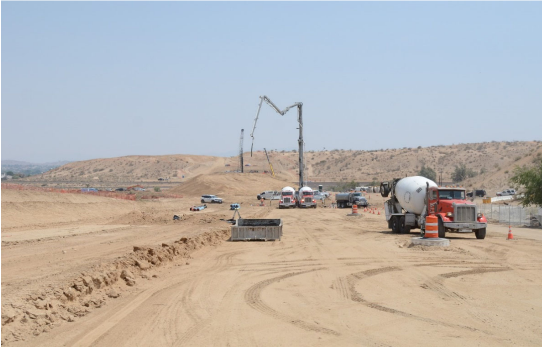
The start of placing many cubic yards of concrete for the bridge.
