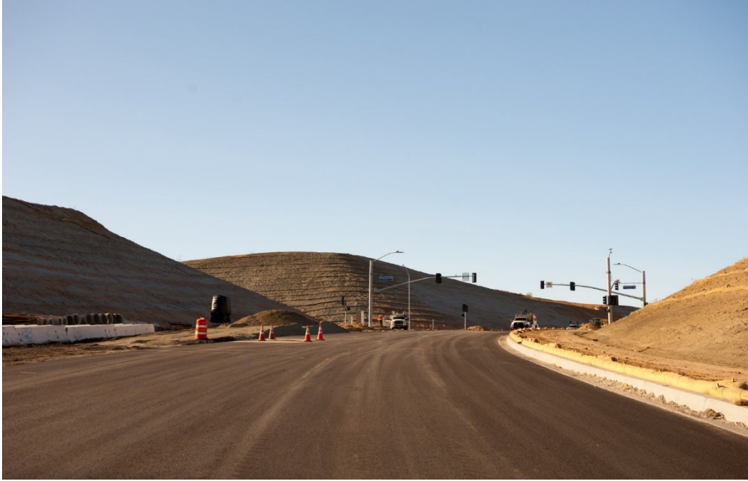
Roadway excavation showing the 60 foot cuts and starting to pave the roadway
