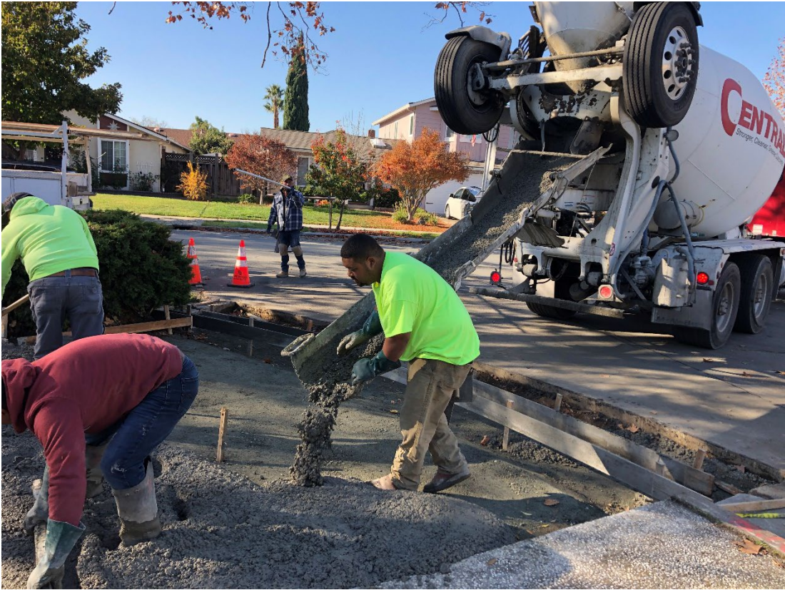
Ramp construction with the crew placing first ever low-carbon CO2 concrete in San Jose.
